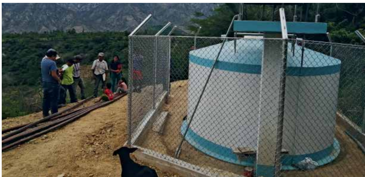
Nimpana chlorination system
