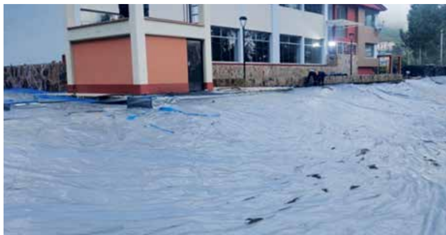
Key: Rapid cover installation to control landslides in the Gran Pajaten Library sloping walls.
