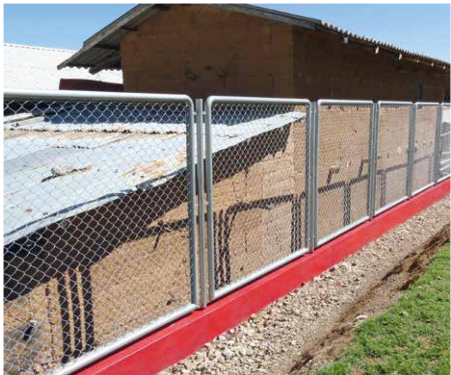
Key: Installation of metallic fence in Jorge Chavez Dartnell School N.80854 in Chuquitambo Community, Pataz District and Province, La Libertad.
