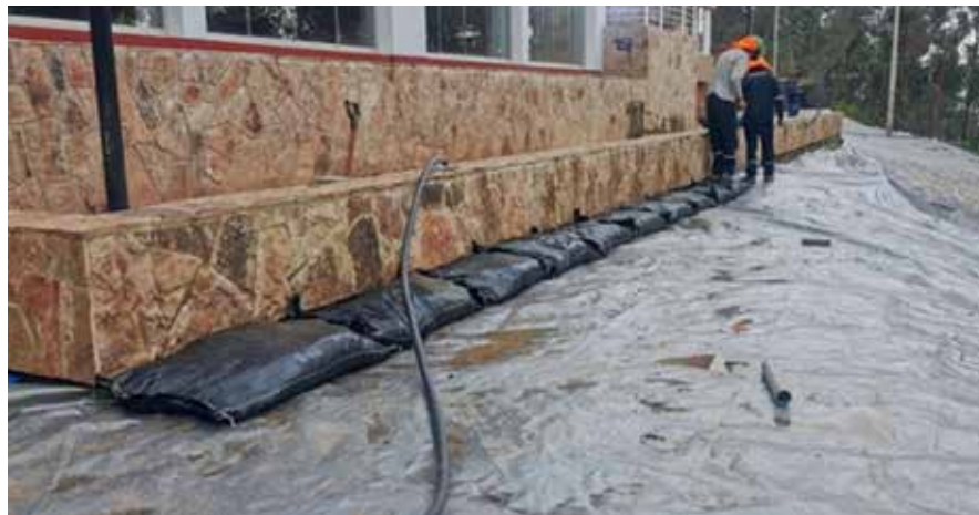
Key: Rapid cover installation to control landslides in the Gran Pajaten Library sloping walls.
